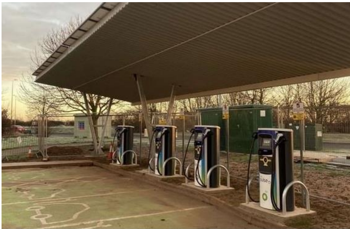
Figure 9: Gamston Community Hall Solar Electric Charging Hub
