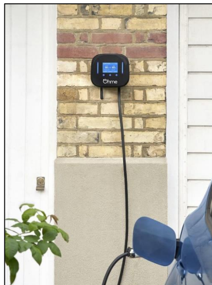
Figure 7: Example of new build EV charge point
